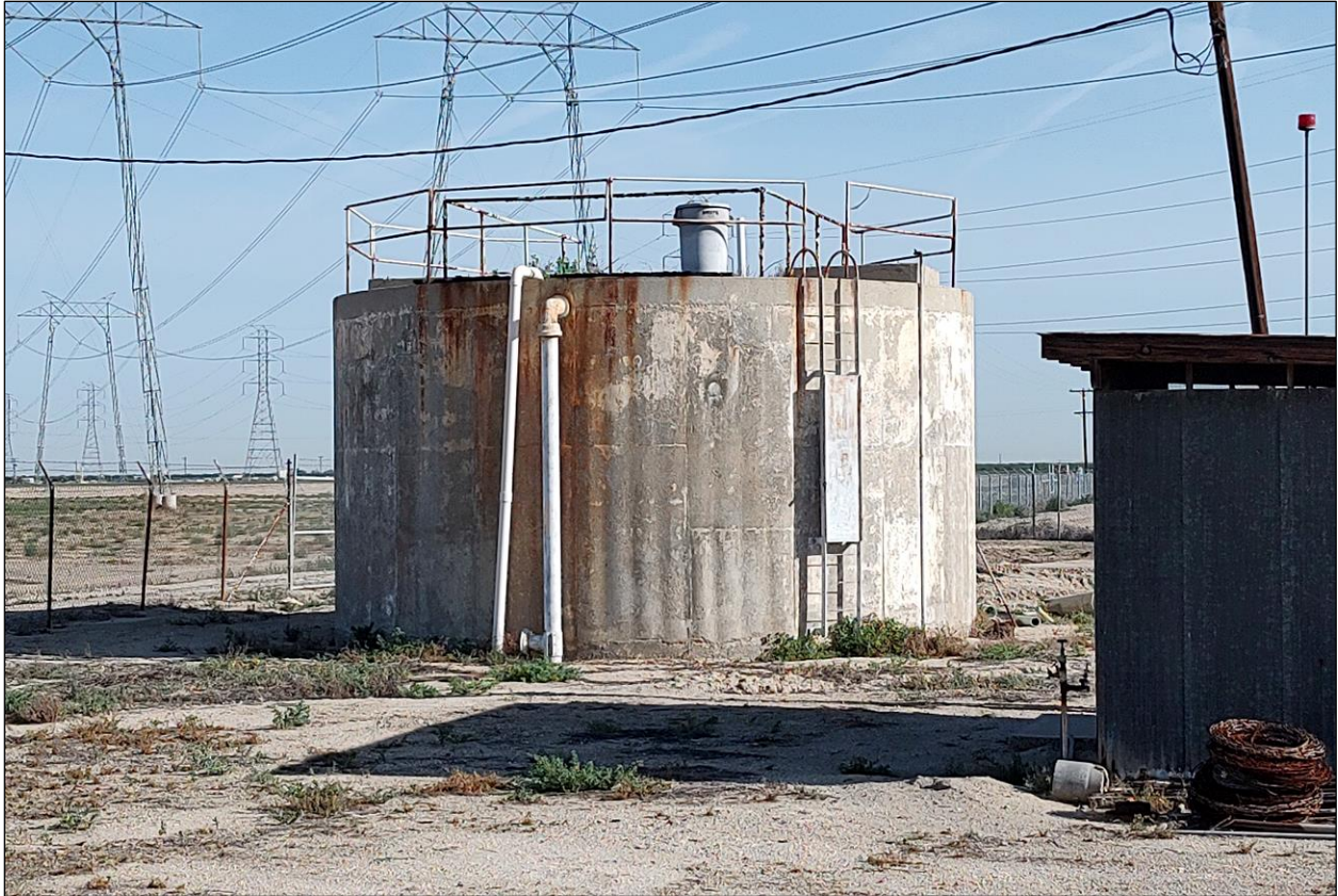
Figure 12. Imhoff tank and corrugated metal shed at Buttonwillow WWTP (Site 3856-4H). (Photograph taken on May 5, 2022; view to the northwest)
