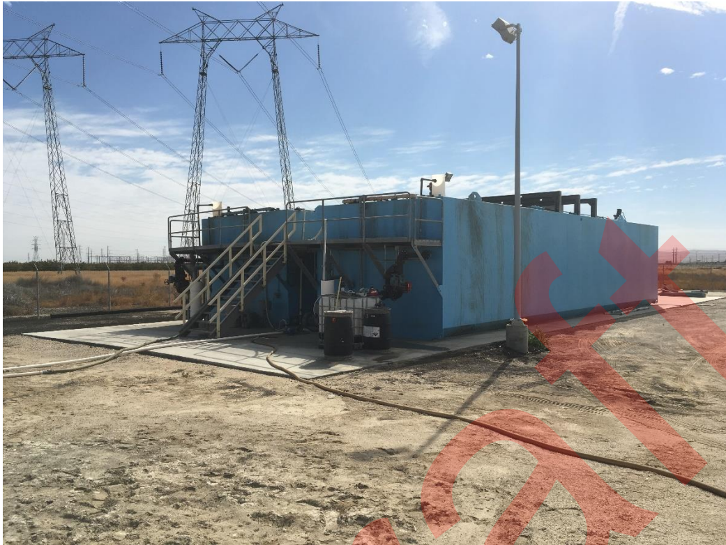
Figure 3-2 WWTP- Bio-Wheel Membrane Plant
