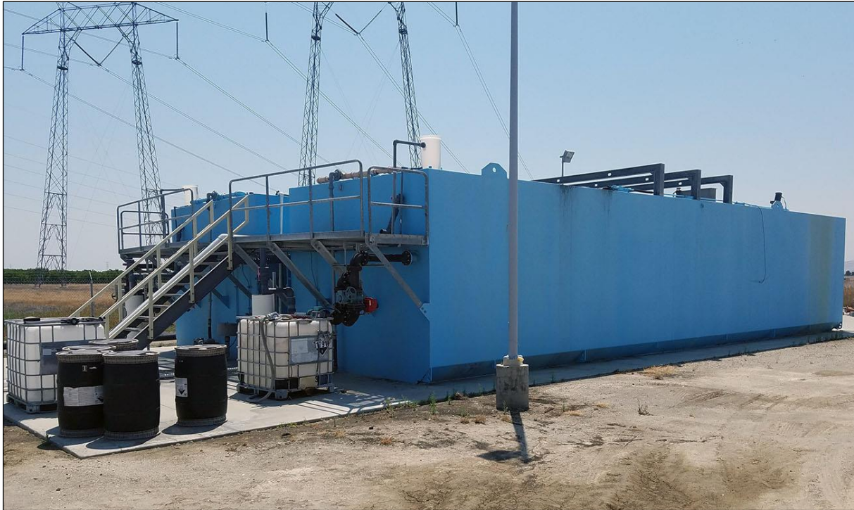
Pre-engineered modular biological treatment systems installed in 2010; view to the southeast
